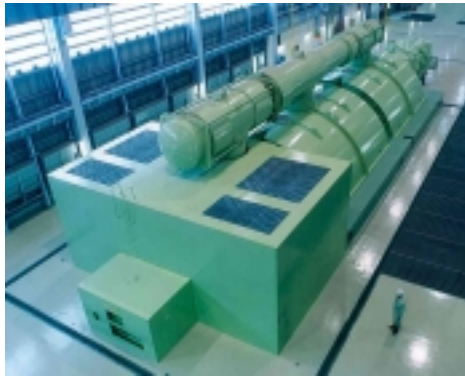
Fig.2 Tomato-Atsuma No.4 Steam Turbine Generator
